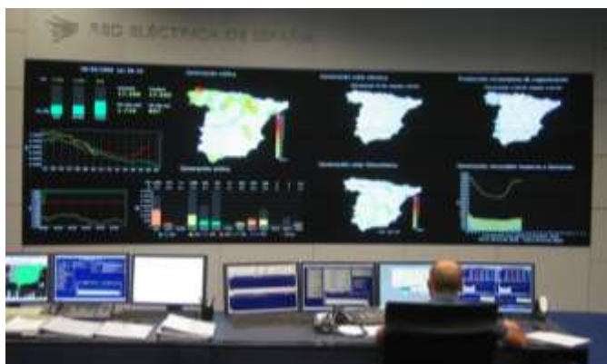
Figure 29 Control Centre of Renewable Energies
